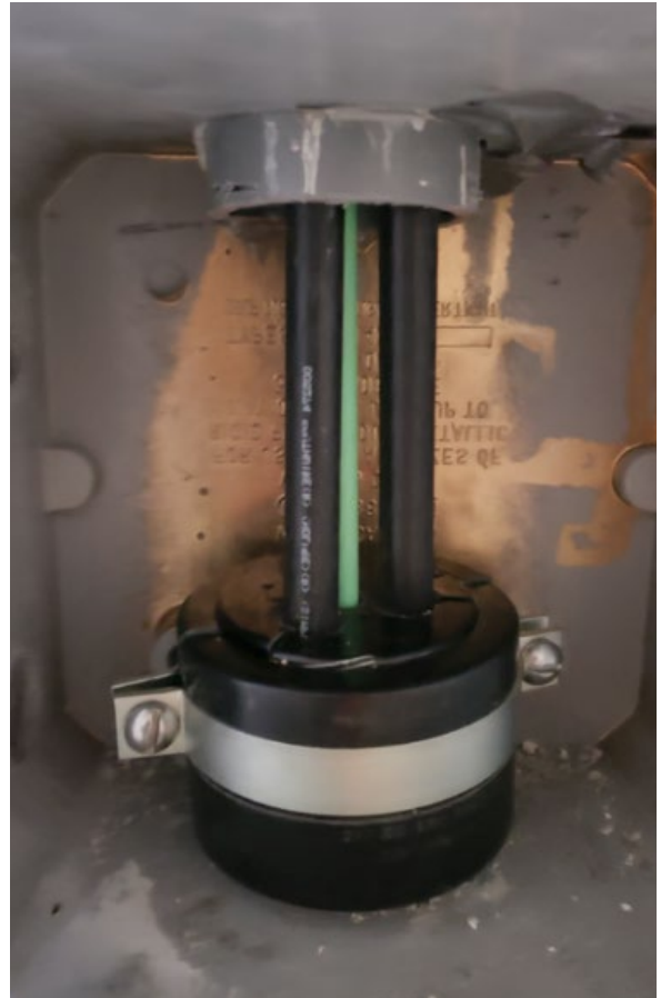
FIGURE 1: Wedge type support within an access box
