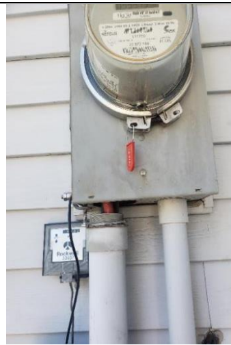
Picture #2 CI Duct & DO Conductor (Barrier) e.g. detached duct
