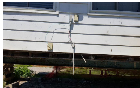
Picture 2: Example of breaking of the ground wire and exposed branch wiring
