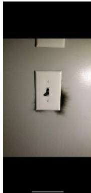
Picture 1, Damage due to Arcing
