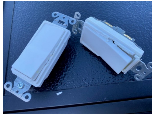
Picture 2, Deterioration Damage to Switch
