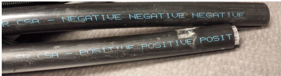
Photo F2 – Example of the required marking to identify polarity
