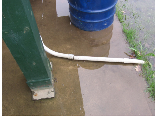
Photo F2 – Improperly protected conduit (Damaged)
