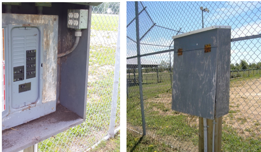
Photo F3 – Accessible and Deteriorated Enclosure
