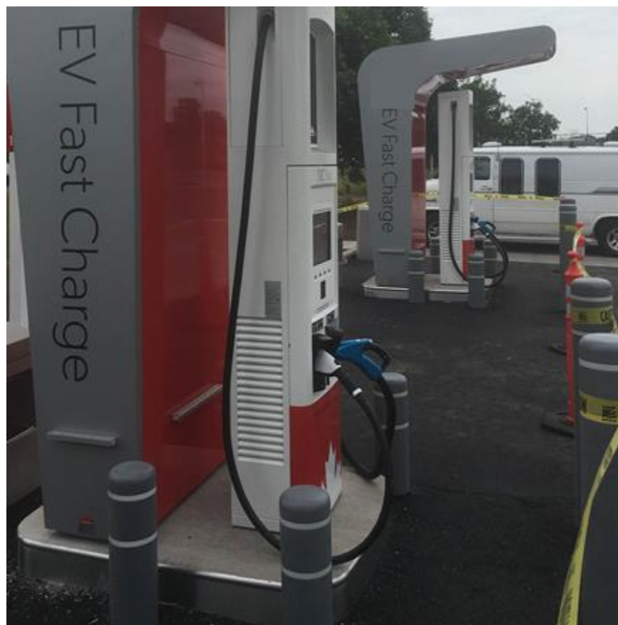
Photo B1 – Multiple DC charging posts fed from a main power cabinet
