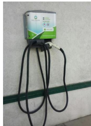
Photo B3 – EVSE protected by height
