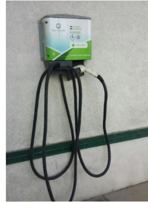
Photo B4 – EVSE protected
