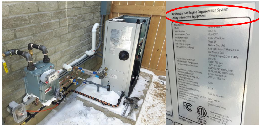
Photo B2 - Example of residential co-generation system and nameplate label
