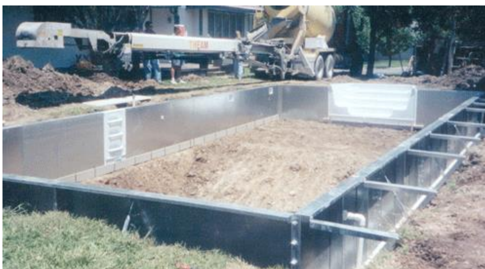
Photo B2 – Metal pool with fibreglass stairs and pool reinforcing brackets
