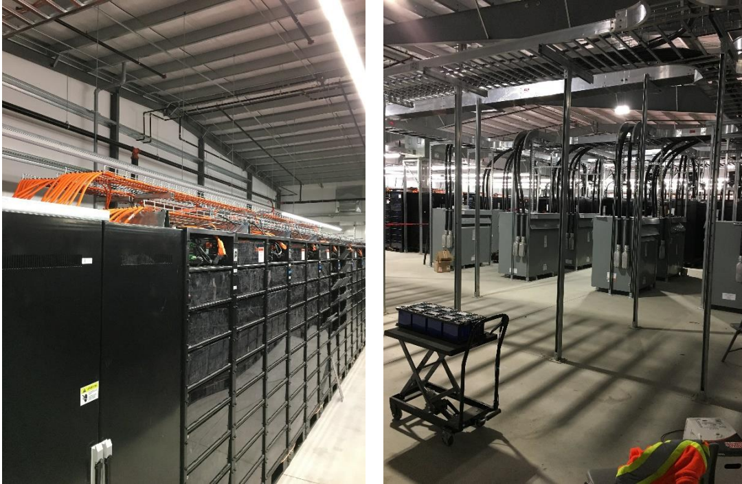
Photo B1 – Example of an ESS
