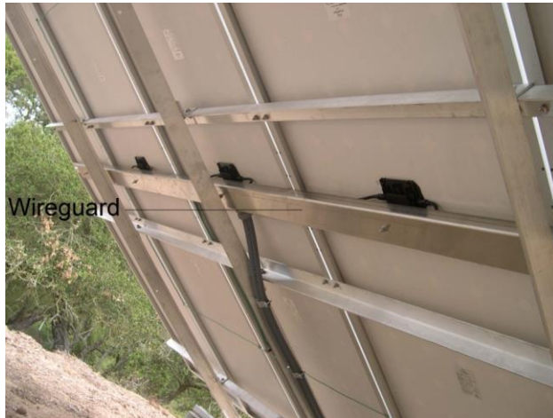
Photo B6 – example of using physical barrier around wiring
