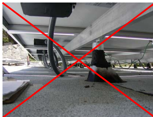
Photo B2 – Unacceptable cable support
