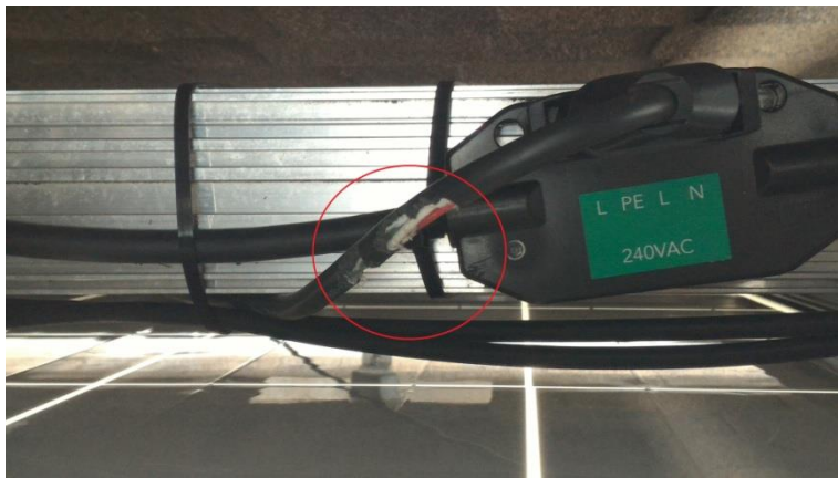
Photo B3 – Examples of rodent damage
