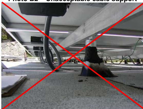
Photo B2 – Unacceptable cable support
