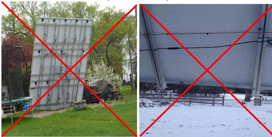
Photo B5 – examples of non-compliant installation
