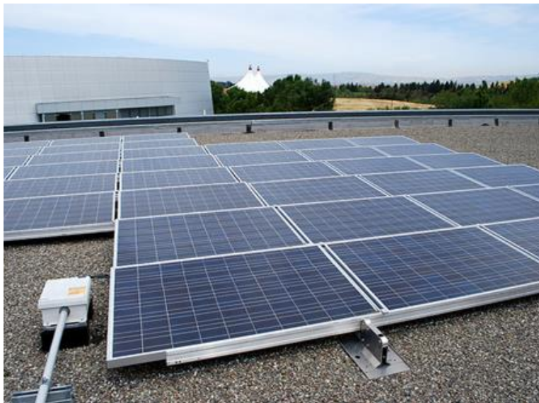
Photo B1 – Combiner box
