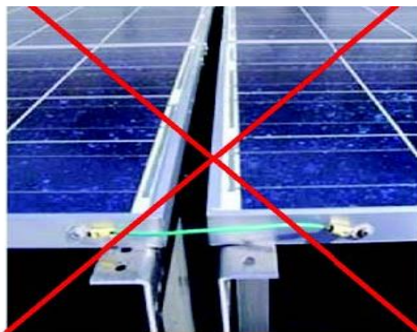
Photo B1 – Unacceptable bonding conductor connection
