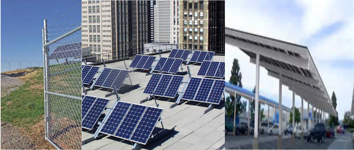
Photo B1 – Examples of PV source and output circuits considered not accessible to the public
