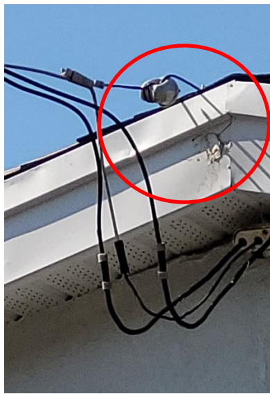
Photo B1- Point of attachment pulled away from the fascia
