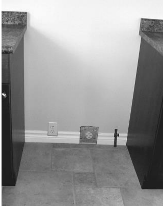
Photo B1 – Code compliant installation of electric and gas range receptacles
