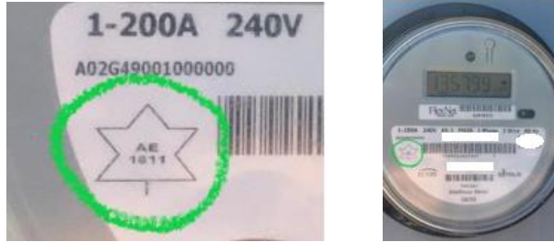
Photo B2 – Socket sub meter
