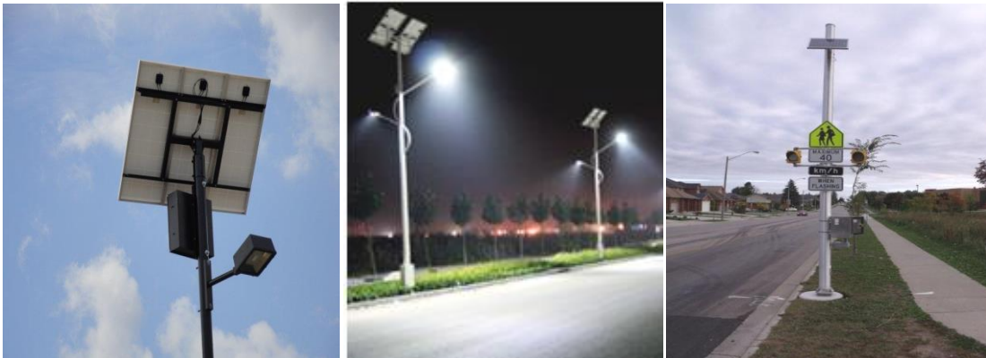
Photo B1 – Example of standalone, pole mounted, solar powered, LED luminaires and flashers
