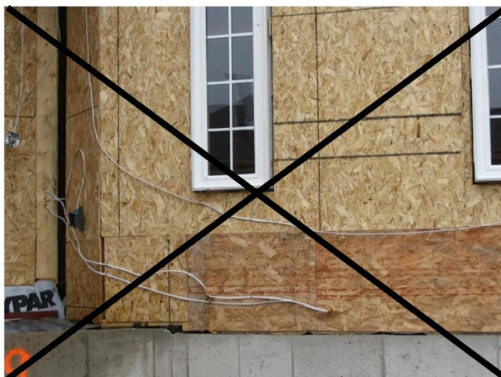
Photo B5 – Installation of NMSC between exterior brick and sheathing; non-Code compliant installation
