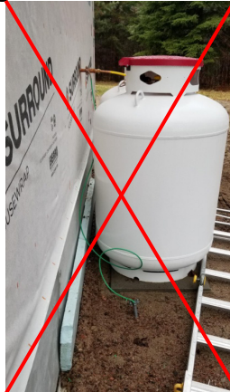
Photo B1 - Example of gas line bonded to a separate ground rod
