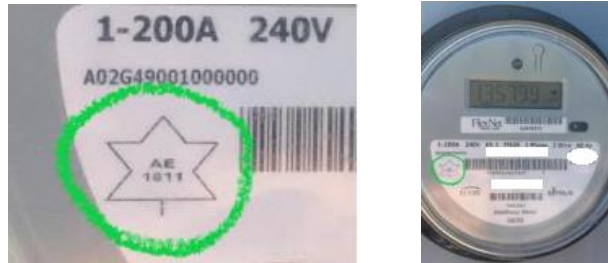
Photo B2 – Socket sub meter
