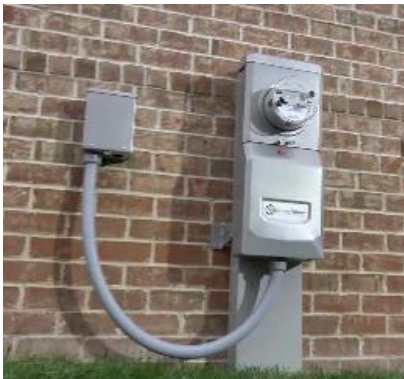
Photo B3 - Meter-mounted transfer switch
