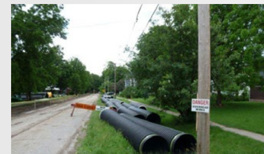
Figure 1: "Danger Overhead Wires" signs posted and barrier blocking traffic.
