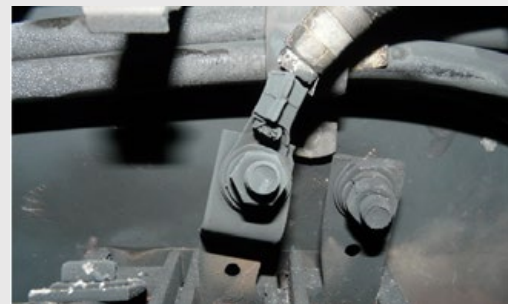
Figure 1. This depicts the remainder of damaged buses which had been energized while Electrician A was attempting to remove the cables behind them.
