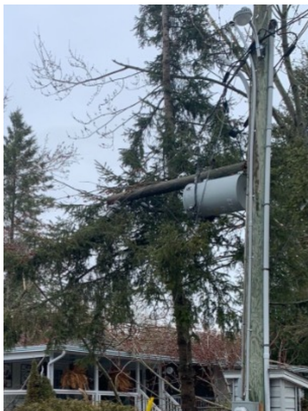
A fallen tree damaged a transformer and strained powerlines on a residential utility pole, creating a dangerous situation
