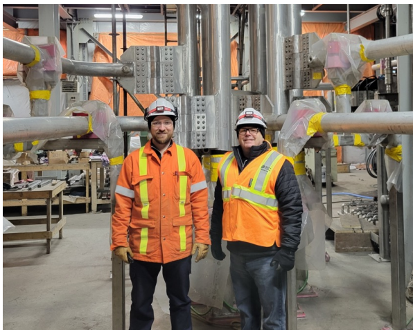
ESA inspectors stand in front of water-cooled aluminum conductors that power the furnaces
