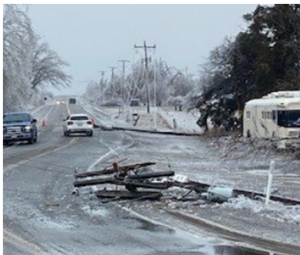
Following the ice storms, hazards like downed primary lines and damaged transformers needed to be addressed quickly
