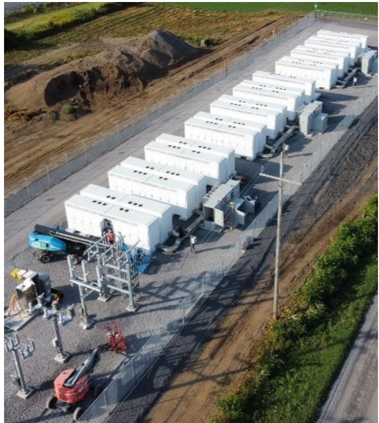
The North Glengarry Battery Energy Storage System
