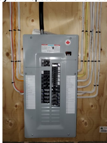
Ready for Inspection: Panel Labelling
