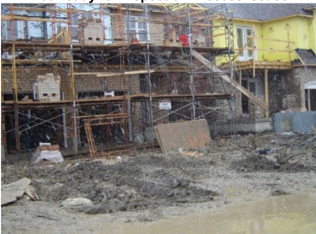
Not Ready for Inspection: Access Issues
