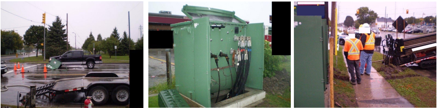
An ESA case involved a directional bore operation at a small plaza
