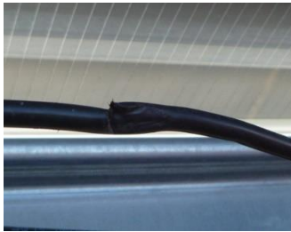
Damaged PV cable
