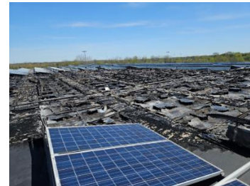
Fire-damaged solar panels
