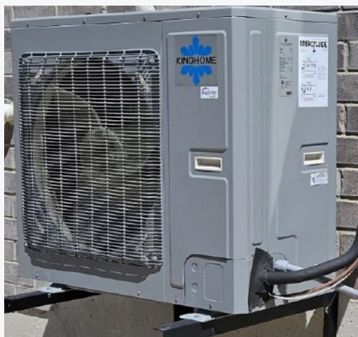
Heat pump for space heating/cooling
