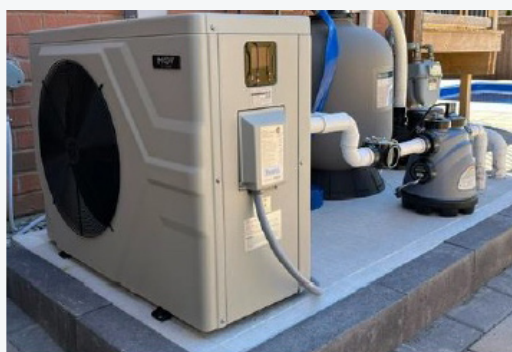
Heat pump for pool heating
